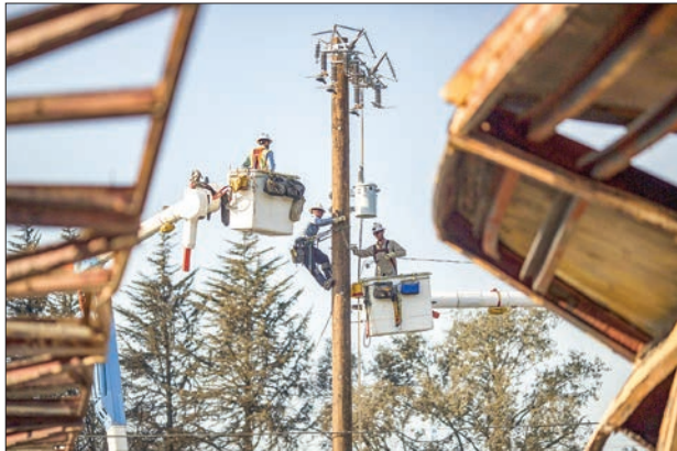
Pacific Gas and Electric Company crews work to restore power near fire-damaged Cardinal Newman High School in Santa Rosa, California on October 14, 2017. PHOTO: DAVID MCNEW / GETTY IMAGES / AFP/FILE
