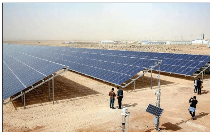
A general view shows part of a new 15 million euro solar plant, funded by the German government, that emits some 12.9 megawatts during its official inauguration at the Zaatari refugee camp on 13 November 2017. PHOTO: AFP
