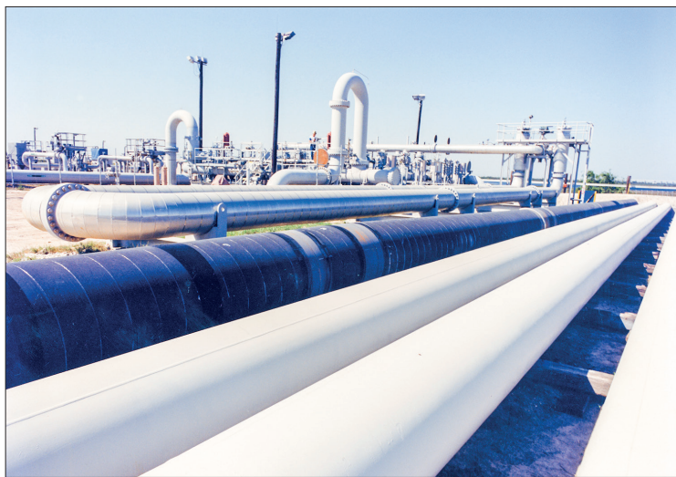
An undated photo provided by the Department of Energy shows crude oil pipes at the Bryan Mound site near Freeport, Texas. PHOTO: DEPARTMENT OF ENERGY/FILE
