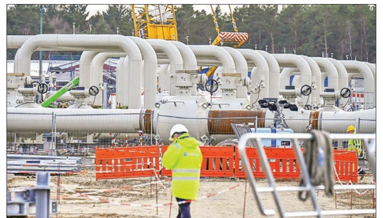
If Russia invades Ukraine, the United States wants to block the opening of the new $12 billion Nord Stream 2 pipeline that is to carry natural gas from Russia to Europe and earn Moscow billions of dollars each year. A worker walks at the construction site of the Nord Stream 2 gas pipeline in Lubmin, northeastern Germany. PHOTO: AFP / TOBIAS SCHWARZ
