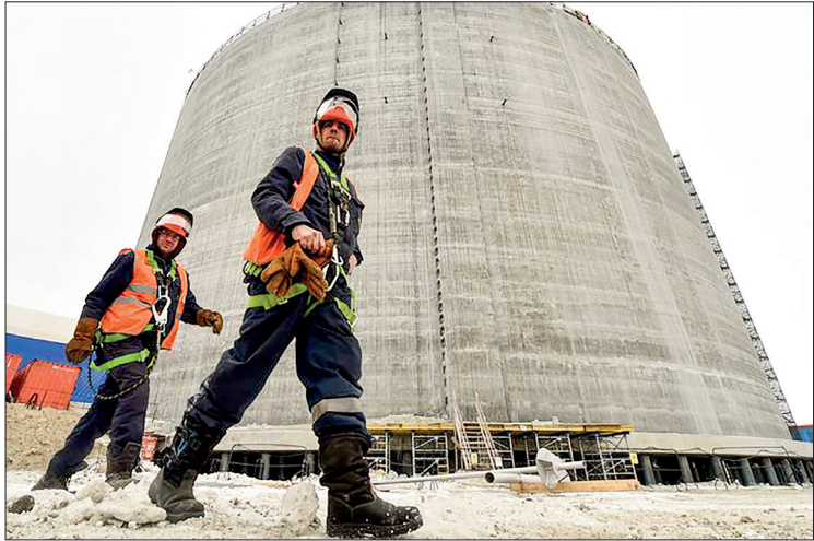
A liquefied natural gas plant being built on the Yamal peninsula, an Arctic region of Siberia that's a key Russian oil-and-gas region. PHOTO: KIRILL KUDRYAVTSEV/AFP
