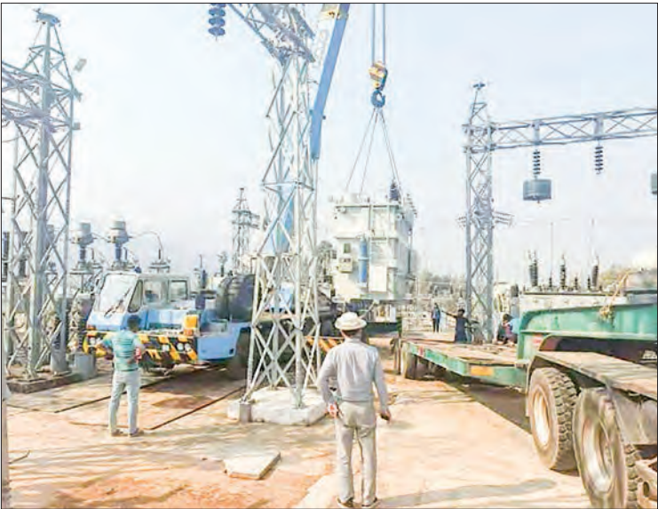
This photo features one of the electricity distribution stations.
